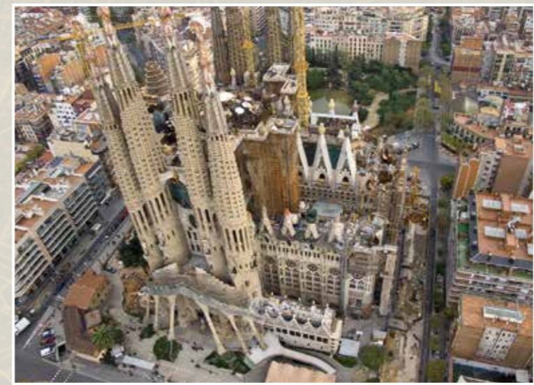
Aerial view of the tunnel works Sants-La Sagrera next to the building of the temple La Sagrada Familia.
